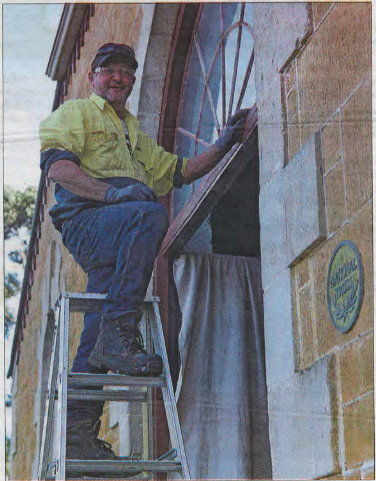
HISTORY RESTORED: David Marshall restores the timber frame of the iconic arch window at the Glencoe Woolshed. Pictures: BRITTANY DENTON
